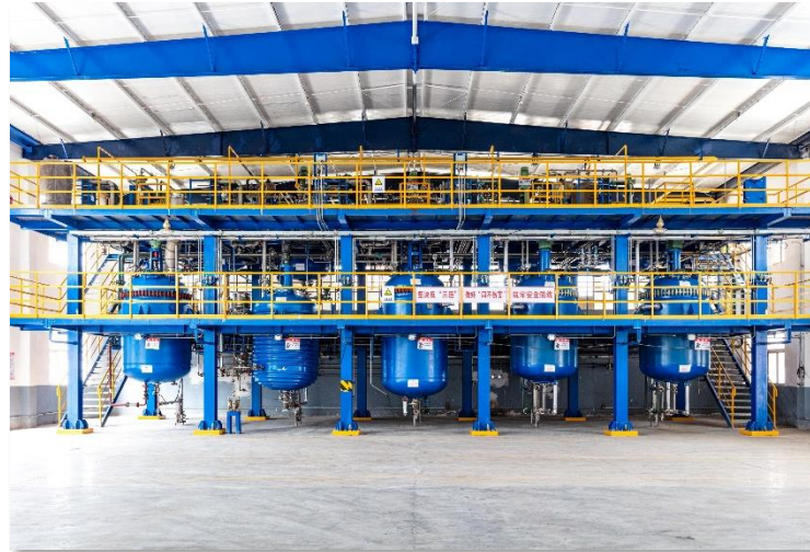
Advanced Manufacturing Equipment
